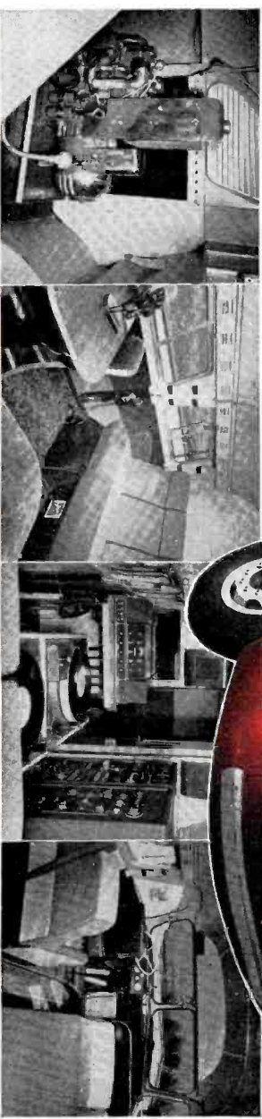
2 KW GEN-ERATOR is located in rear compartment of unit converted from 29-passenger transportation bus by WKY engineering staff.
